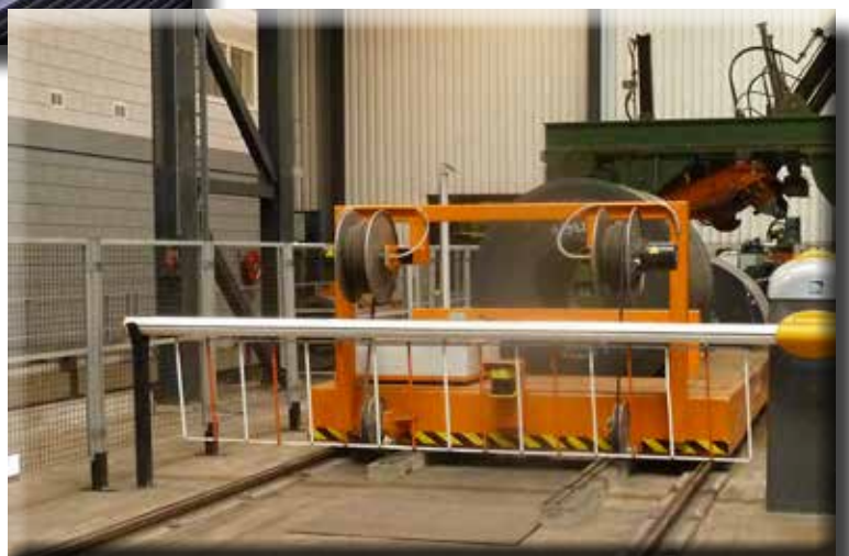
AV40 cable reels for feeding and controlling of a transfer cart and machines
